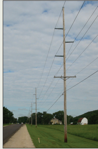
69-kV/115-kV transmission structure with distribution underbuild
