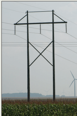
230-kV/345-kV H-frame transmission structure
