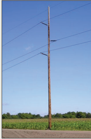
69-kV/115-kV transmission structure
